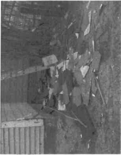
Improperly removed asbestos from home renovation project.
