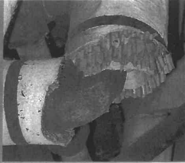
Damaged asbestos pipe insulation.
